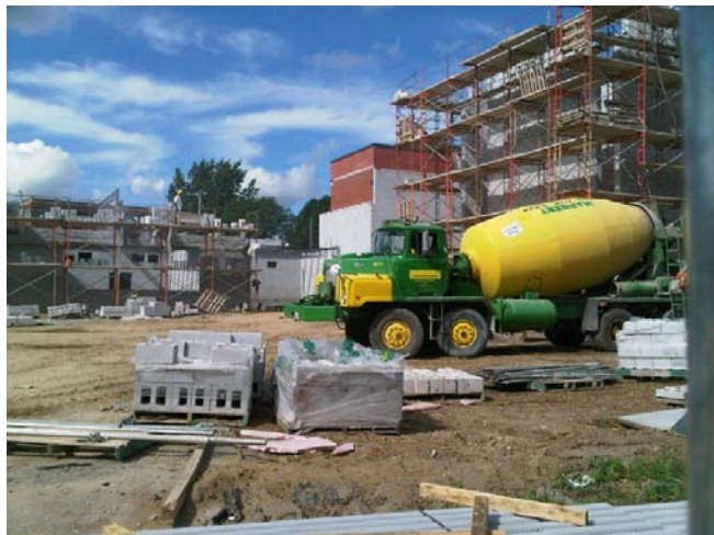
The students & staff of Monsignor Gleason / St. John CES are eagerly anticipating the re-built St. John CES as construction moves along nicely on Strange St. in Kitchener.
